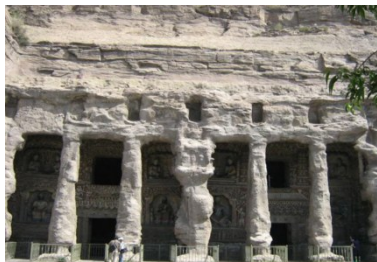
(c) Rock pillars exposed to the water-rock cycle [57]
