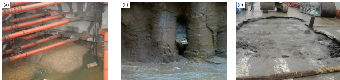
(a) Leakage of groundwater and sand
